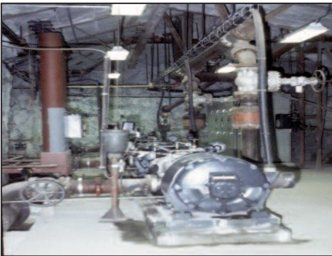
Pump on the 1850-foot level of the West Shaft.
