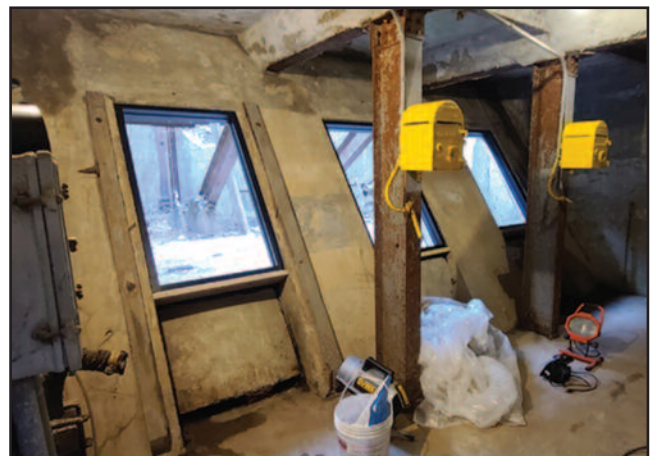
The historic East Shaft is visible through three, newly installed, tempered glass frames. The viewing room will receive rubber-vinyl flooring and will be easily accessed via the existing stairway leading down to the GeoTech Center.
