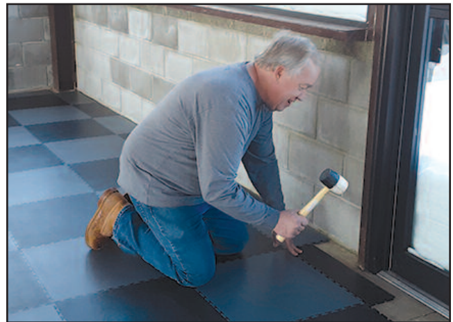
Tour guide and maintenance man, Ken Daubert, installs a new hi-tech floor in our pavilion. The interlocking/dovetailed tiles are free-floating for expansion and contraction, and are gently hammered into place. It is amazing how much difference a new floor makes in improving the overall environment.
