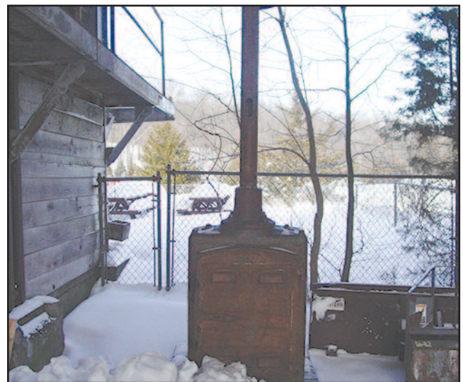
The cabinet base and mast for the block signal have been stripped of paint and await power-washing and painting. They are protected from the elements under our conveyor tower for now. This unit will be set on a new concrete pad, with electricity fed from below into the cabinet to make the signal fully operative.
