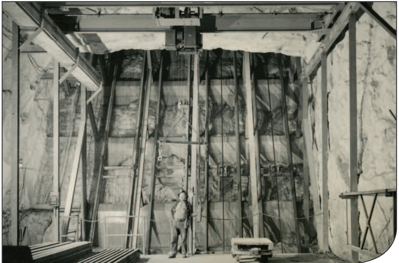
Adit shaft station, circa 1956, still under construction in this photograph; completed in 1958. New steel tracks are visible on the floor, soon to be lowered and installed in the shaft. The cages rode on these rails down to 1920 level. The compressor pipes and the main water pipe that carried the pumped water from the mine are not yet installed. They will be in the far left compartment. The overhead travelling hoist is still in place to this day, although not operable. [Ed. note: for information on an exciting new project at Sterling Hill, an exhibit with a motorized man cage at the shaft station, see the Message from the President in this issue.]
