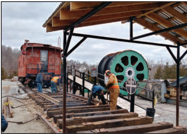
The work that would have taken us weeks was professionally accomplished in a mere three hours by the NYS&W railroad crew. Over 80 feet of additional track has now been added to our new railroad pavilion.
