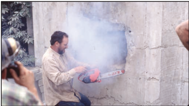
Bob Hauck using a chain saw to cut through timbers behind the concrete plug.
