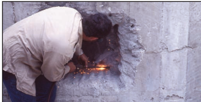
Bob Hauck using a torch to cut the drill steel that was used by the New Jersey Zinc Company as rebar in the concrete plug.
