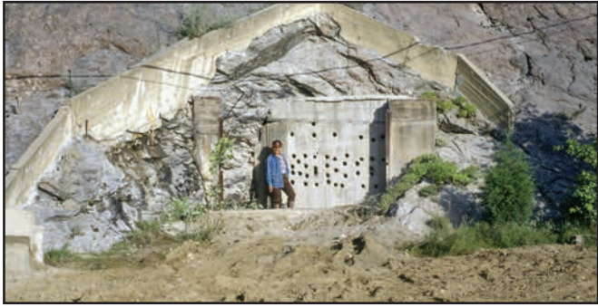
John Kolic, standing by the safety exit, with holes drilled for air circulation.
